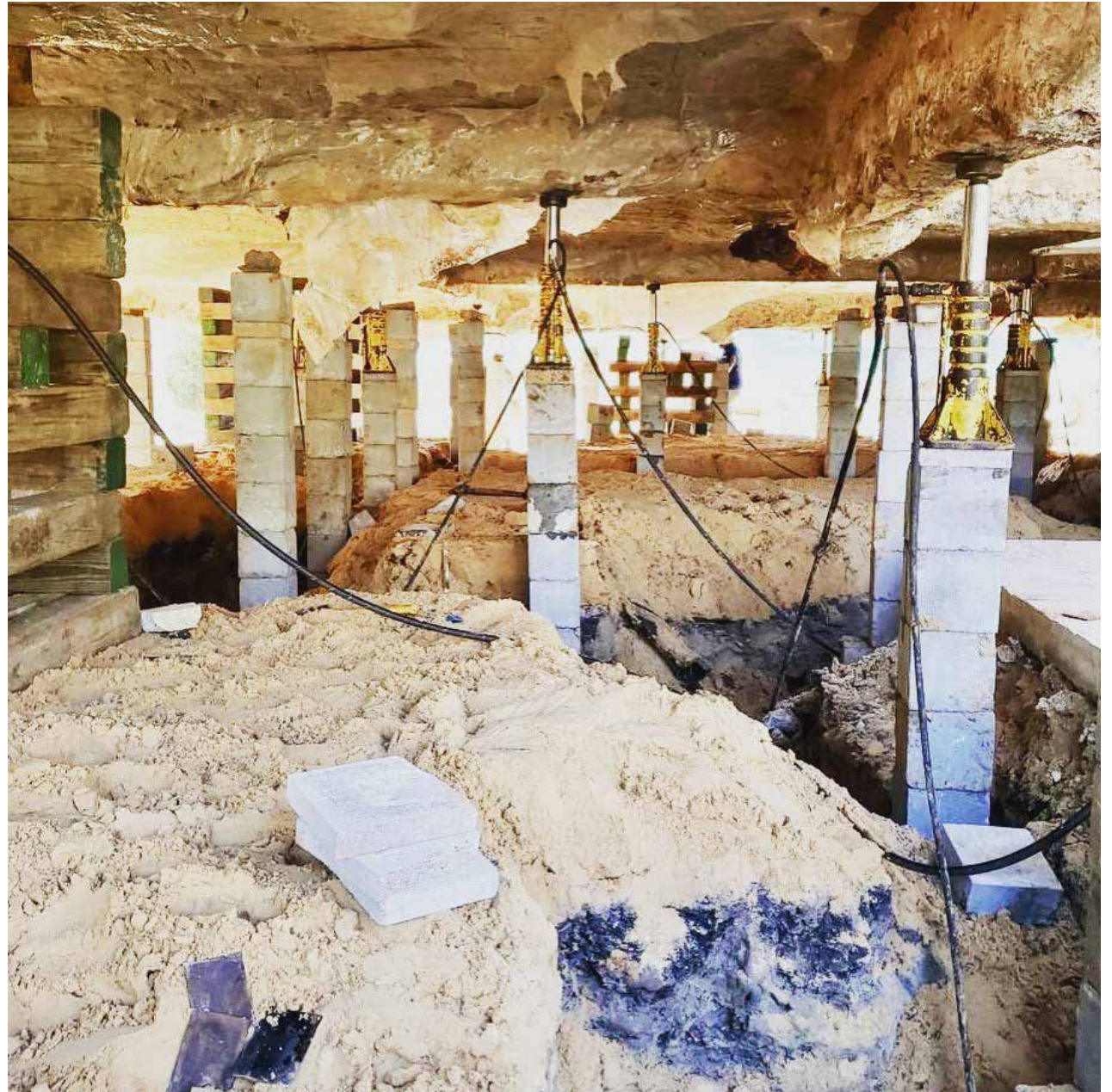
[79] Buildings on a concrete slab can be more challenging to lift. In some cases, as shown in this example, the existing slab can be lifted and still remain the floor for the interior spaces. In other instances, the slab may need to remain at grade, with a new elevated floor structure constructed above. Photo: p3elevation.com
