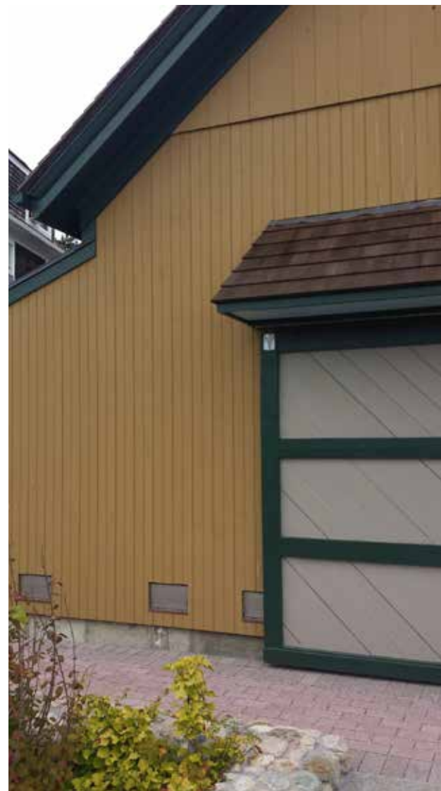
Figure 7: As part of wet floodproofing the building, engineered vents near the bottom of exterior walls are designed to allow water to flow in and out of the building during a flood. This allows water pressure to equalize on both sides of the wall and reduce stress to the structural system. Photo: Jennifer Wellock/NPS
