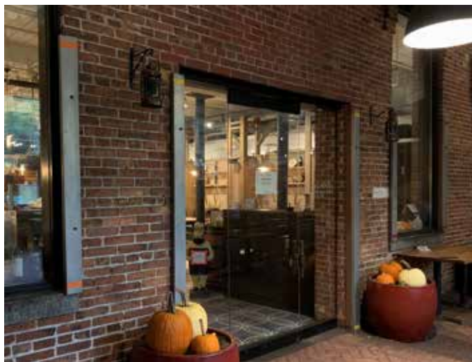
[25] Permanent stanchions at windows and doors in this former industrial mill in Baltimore, MD, are used to attach temporary floodgates to protect openings in the event of a flood. Depending on their size, color, and finish, these stanchions can be quite noticeable. In the case of an industrial property, this may not cause a significant change in historic character. In a different type of building, it is important to ensure that such permanent features blend in and are as visually unobtrusive as possible. Photo: Jennifer Parker/NPS
