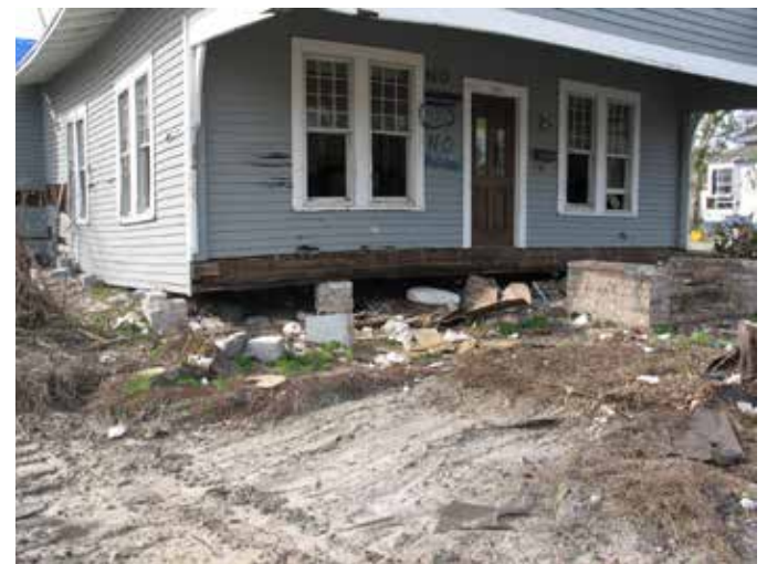
[11] Flood forces are powerful and can result in a building being shifted from its foundation. This historic property in Gulfport, MS, was knocked off of its piers by Hurricane Katrina in 2005. Photo: Jennifer V.O. Baughn/ Mississippi Department of Archives and History, January 26, 2006
