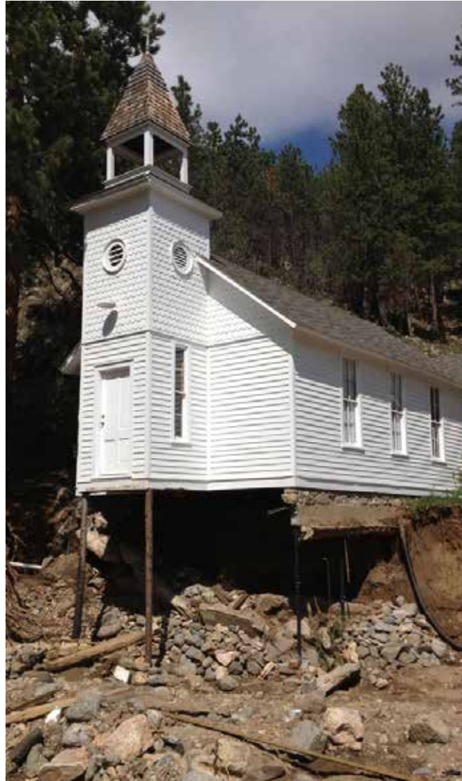
[9] Fast-moving flood waters can undermine a foundation or scour out land around a building. The Little Church of the Pines in Salina, CO, was left structurally compromised after heavy rains caused flooding in the Front Range of the Rocky Mountains in 2013. Photo: Burton Construction burton-construction.com
