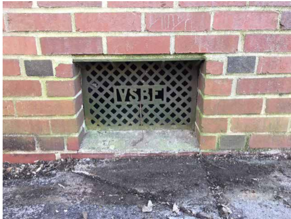
[56] To create a watertight seal around the building, any existing vents or openings below the established flood risk level must be sealed during a flood. Vents that cannot be sealed internally will require an exterior and/or interior cover to keep water from entering the building. Photo: Chelius Carter
