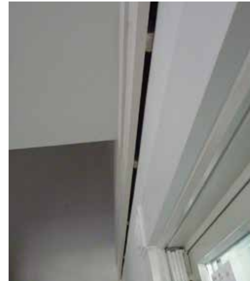
Figure 4: Crown molding covers an opening at the top of walls to allow air to circulate and dry wall cavities after a flood, seen here before the sacrificial insulating foam strip has been applied. Photo: Mary Delaney Krugman, JD, MSHP
