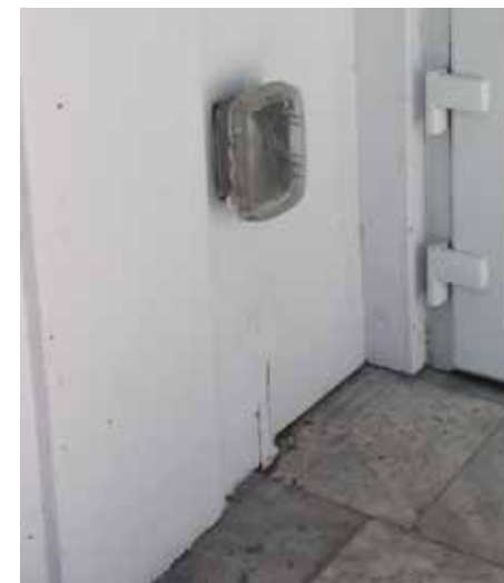
[61] This electrical box is protected with a removable waterproof plastic covering. Alternatively, electrical outlets can be located above the flood inundation level. Photo: Liz Petrella/NPS
