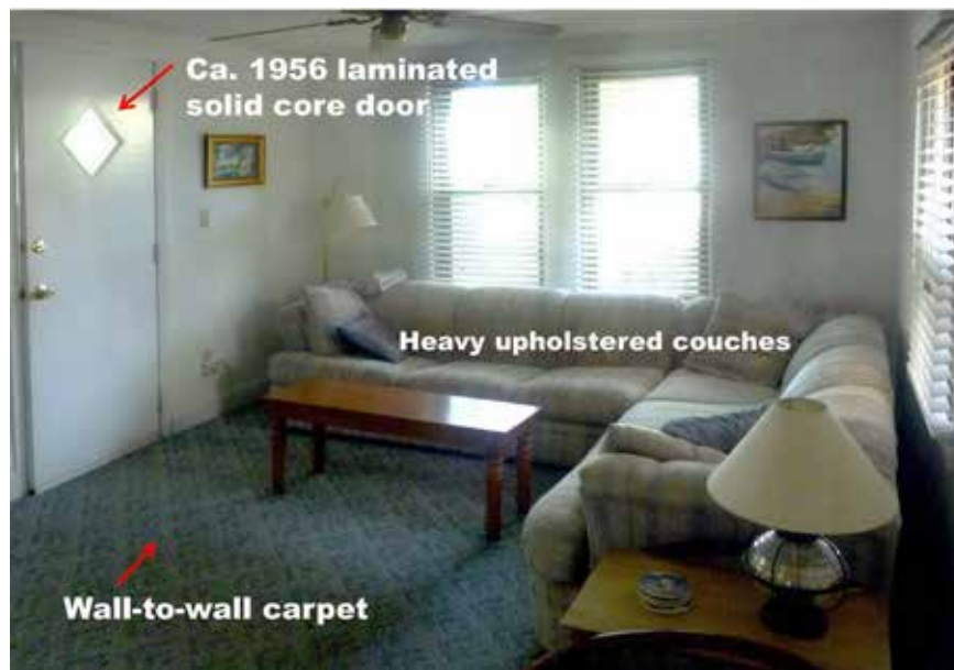
Figure 6: The living room before Hurricane Sandy included non-historic wall and floor finishes. Windows and doors were also non-historic and made of materials that absorbed floodwater, warped, and/or could not easily be cleaned. Photo: Mary Delaney Krugman, JD, MSHP
