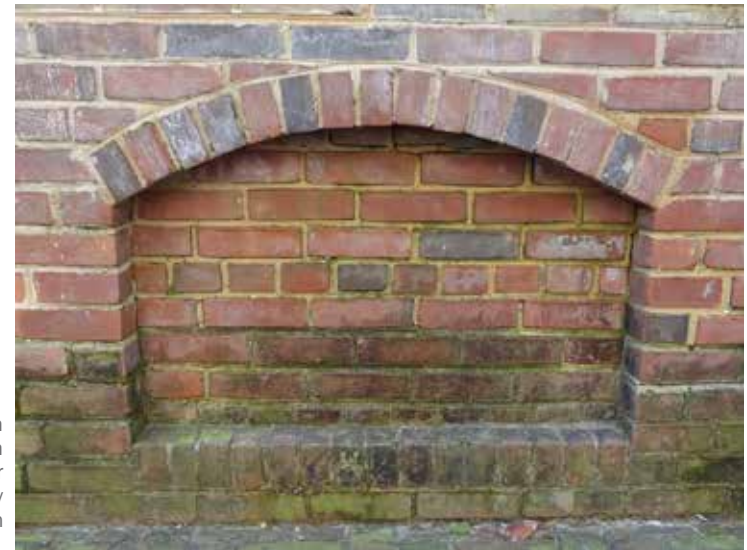
[50] To keep water out of a building, openings on secondary elevations may be permanently infilled with masonry to match or blend in with the walls. Any sills or lintels should be preserved in place, and the masonry infill should be inset to preserve the historic fenestration pattern. Photo: Jennifer Parker/NPS
