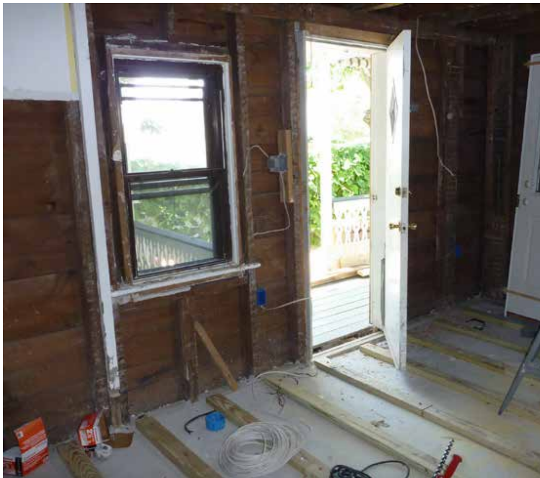
Figure 2: In-progress repairs after Hurricane Sandy. Walls are open to the interior for initial drying. A new concrete structural slab has been topped with treated wood sleepers in preparation for a new flood-damage resistant mahogany floor. Photo: Mary Delaney Krugman, JD, MSHP
