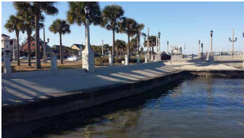
[34] Some flood protection structures are historic, such as this seawall in St. Augustine, FL. The seawall was constructed in sections over time beginning in 1696 near the Castillo de San Marcos. Photo: Jennifer Wellock/NPS
